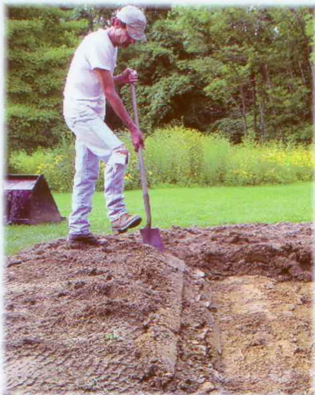
You can dig your rain garden by hand or use a backhoe. If you use a backhoe to dig your garden, avoid driving it on the garden site to minimize soil compaction.
